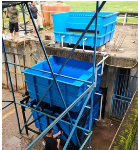
Figure 2. Clean Water Treatment Installation in Sidang Kasiak
